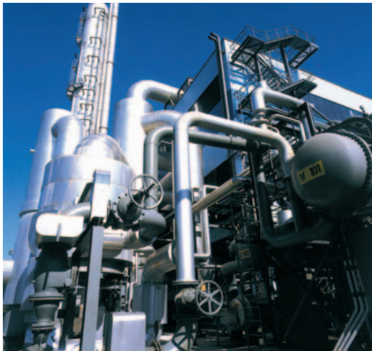
Left: Nitrous oxide removal: The new process, which has until now only run on a pilot plant, is now being implemented in a full-scale plant at Agrolinz Melamin's Austrian location.
