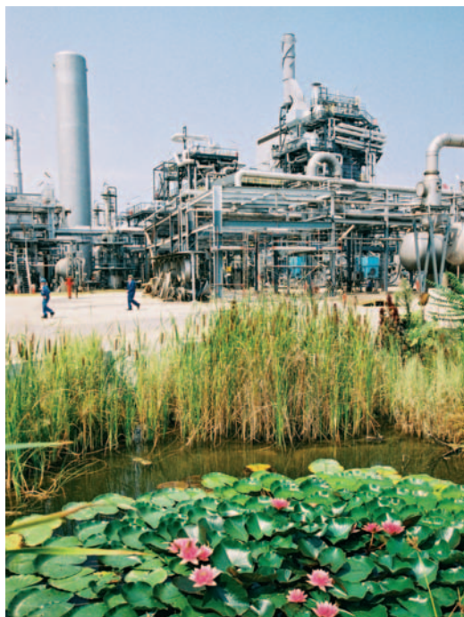
Hydrogen plant commissioned in July 2003, Schwechat refinery.
